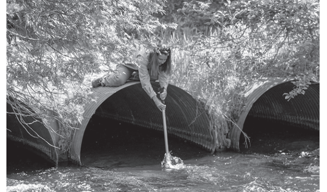
CRA Program Director Kimberly Balke measures the river's velocity at site #WA-5 (Jordan River and Jordan River Road-West). The undersized culverts create a velocity barrier to fish and other aquatic species.
